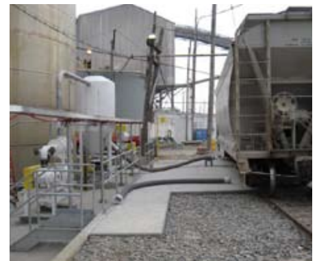
Operators use USS urethane sleeves to quickly hook hoses up to the railcar.
