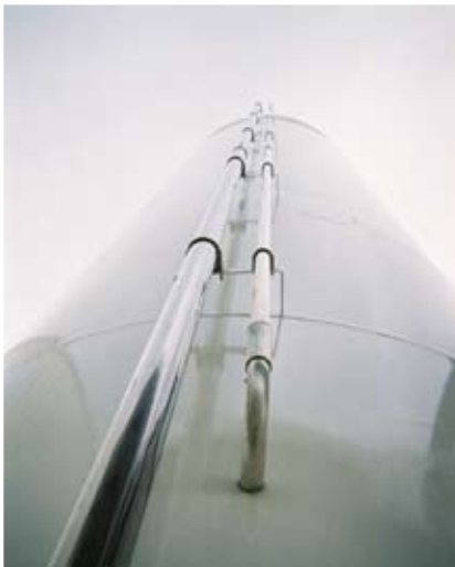
USS designed the entire system from railcar unloading to storage to wet mix tank.
